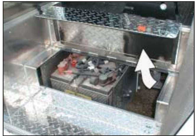
Figure BA-10 Stepwell Battery Access
